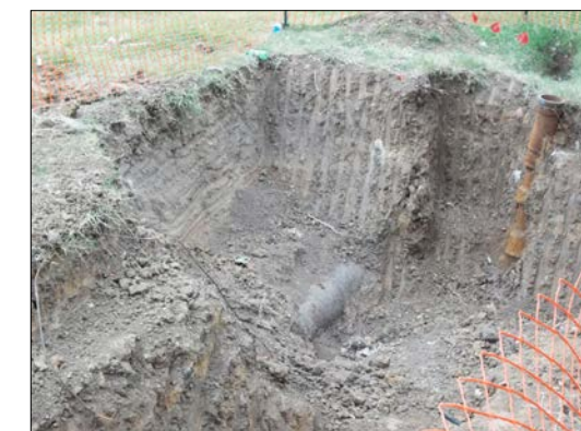
Figure 4. Photos of the site, showing status of work and proving that one can review compliance associated with the ticket.
